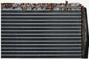
Figure 3: Corrosion on radiator fins
