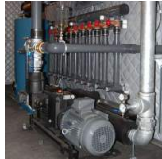
Soil vapour extraction system
