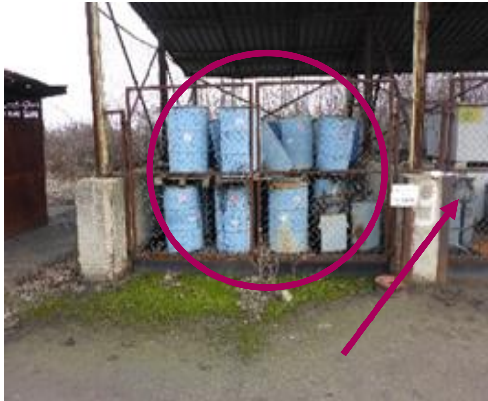
Stockpiles drums with oil containing PCB and electrical equipment containing PCBs
