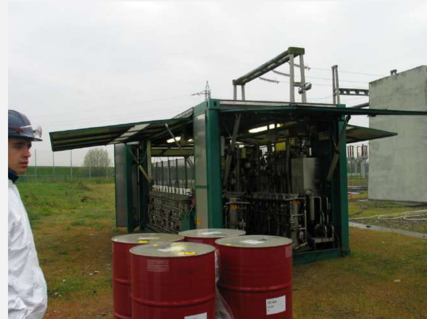
Source: Overview of PCB disposal technologies – Carlo Lupi – UNIDO consultant
